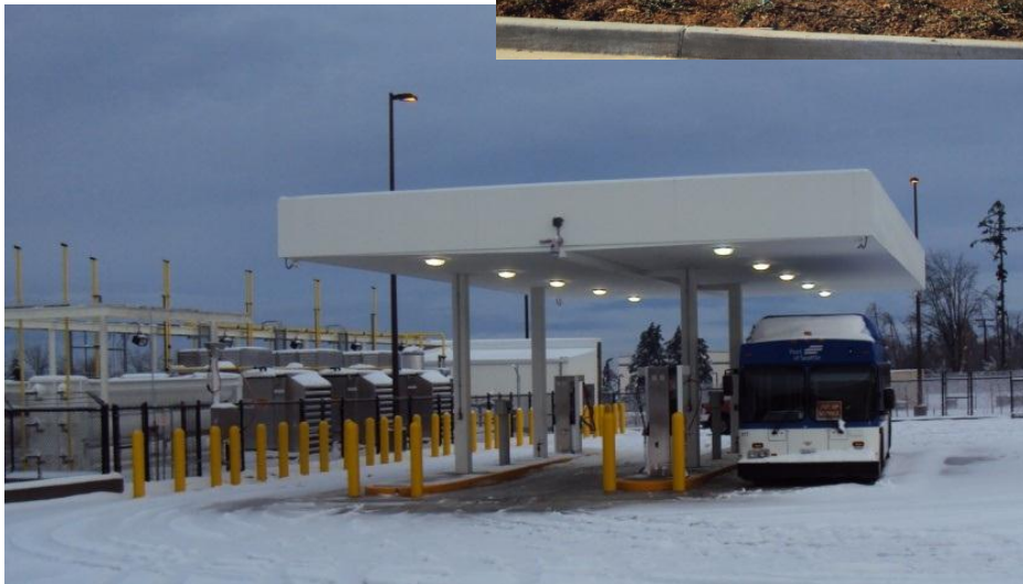
CNG Fueling Facility
